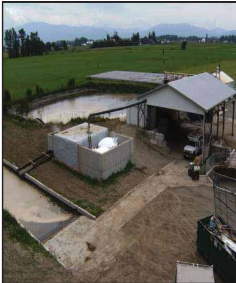
Figure 9: Image of completed system
