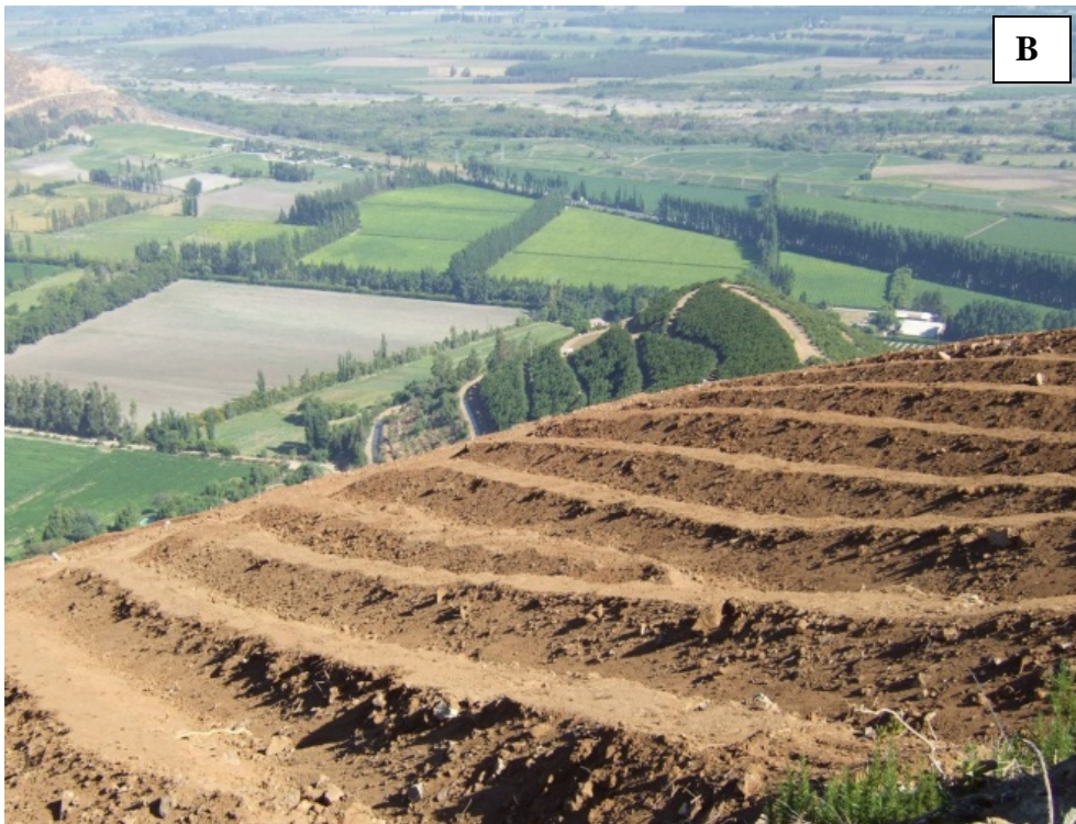
Figures 1A- Hillside after the removal of native vegetation; 1B- Raised berms parallel to the slope, prior to planting avocados.
