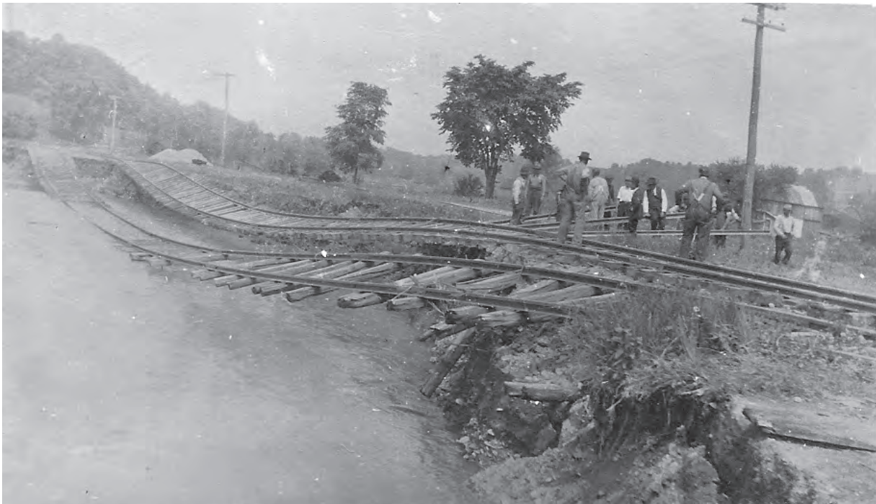
Track crews start to work on a washout near Breesport.
